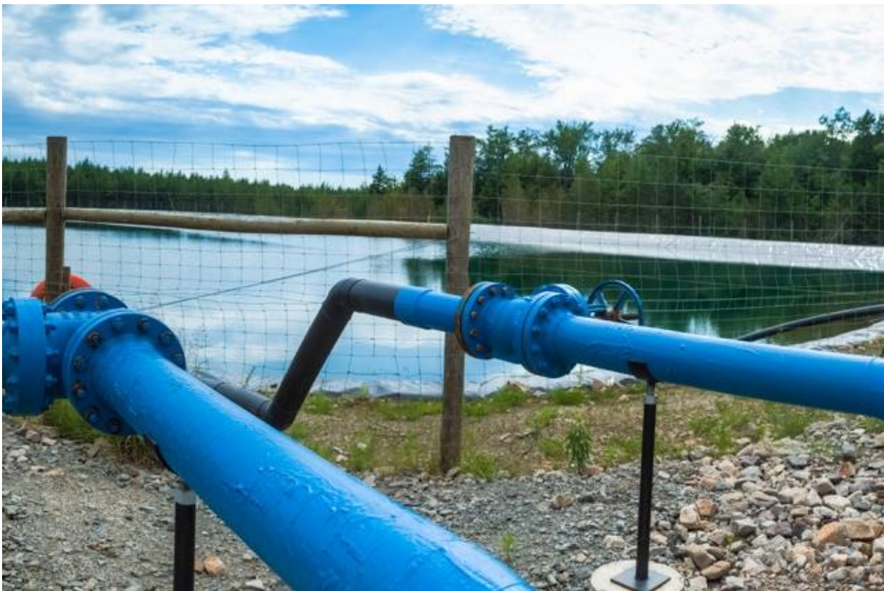
The new desalination method could be useful for cleaning the contaminated water generated by hydraulic fracturing, or fracking source - news.mit.edu
